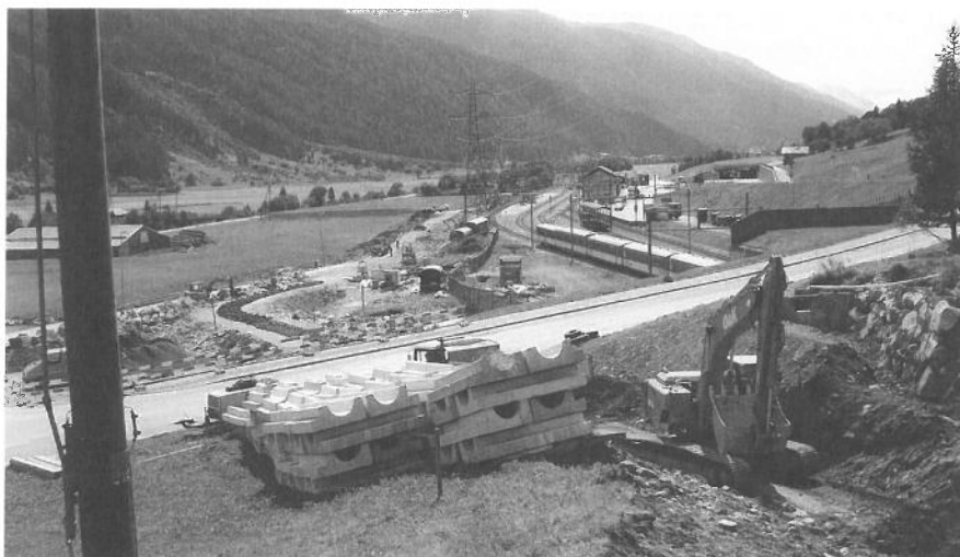
Bauplatz Oberwald (Foto: Peter Studer, September 2009) Chantier Oberwald (photo: Peter Studer, septembre 2009)
